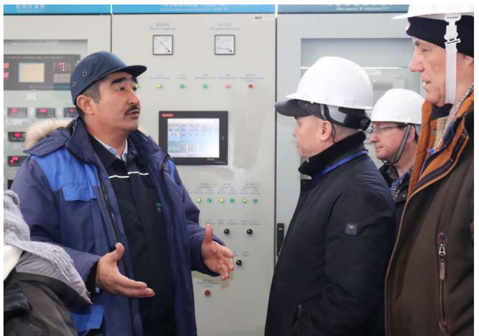
Moynak Hydropower Plant, Almaty, Kazakhstan
