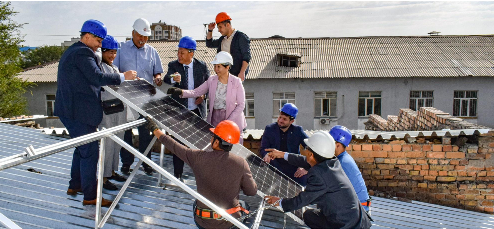
PHOTO: THE USAID POWER CENTRAL ASIA ACTIVITY
